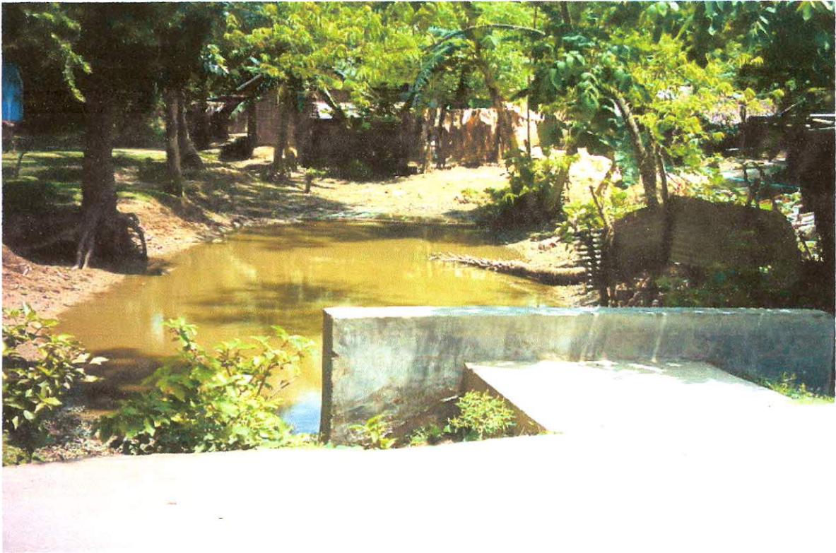
Plate 5: Canal encroachment by settlement
