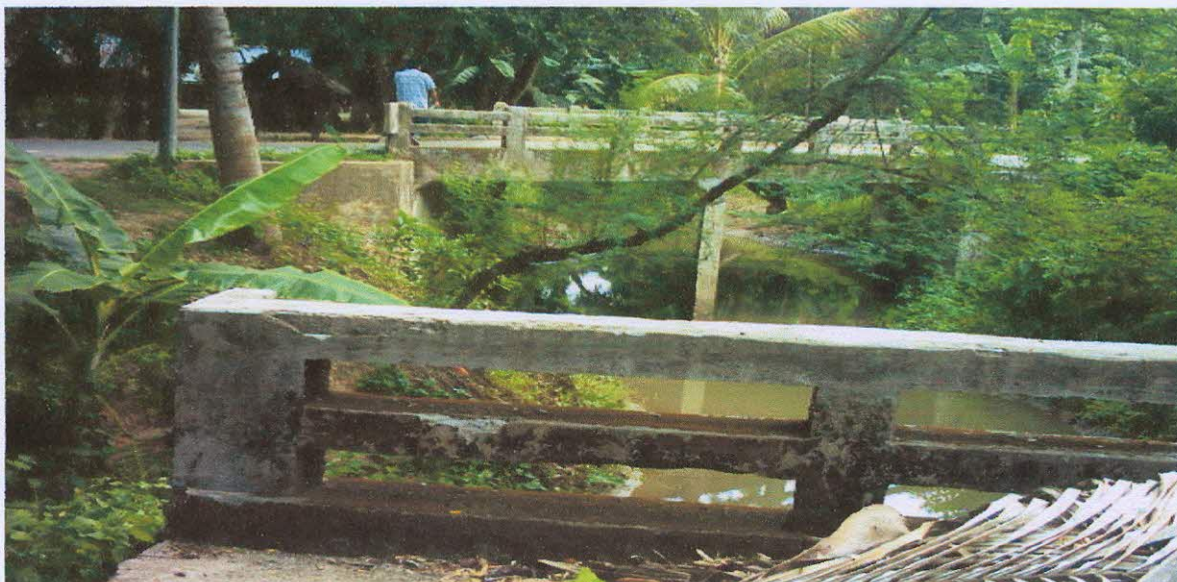
Plate 15: Two culverts were constructed within two years and located at the same point; the photograph was taken from old one
