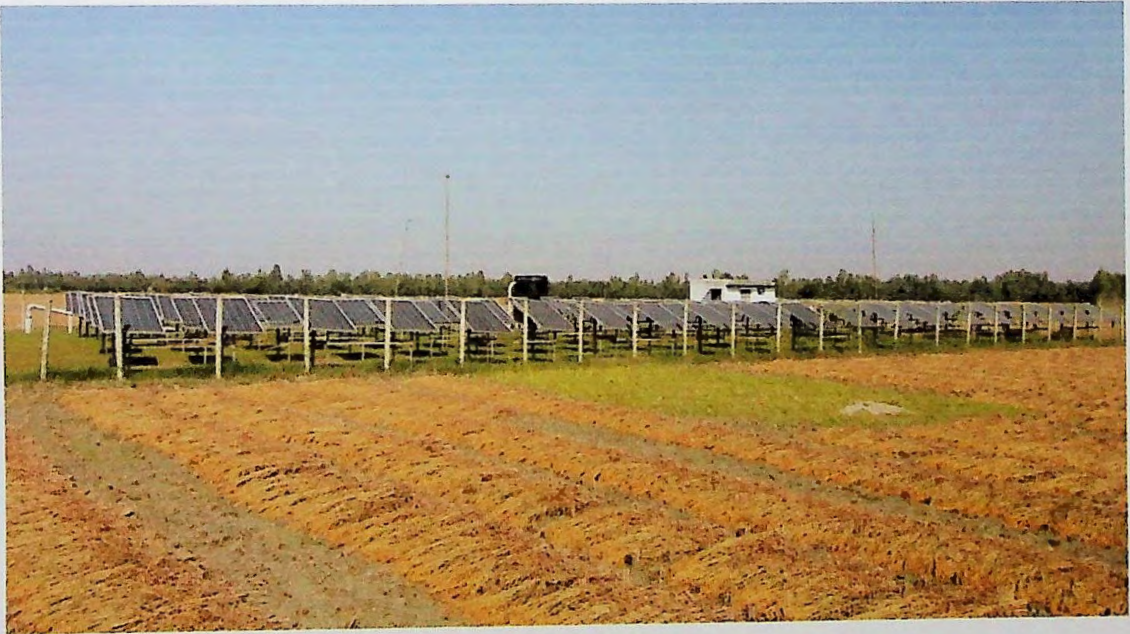
A visited solar irrigation pump in Birganj, Dinajpur
