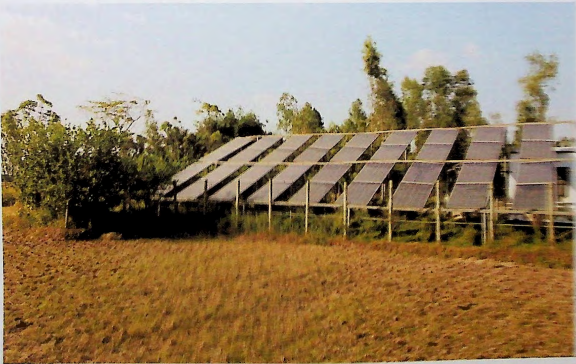
A visited solar irrigation pump in Nandigram, Bogra.
