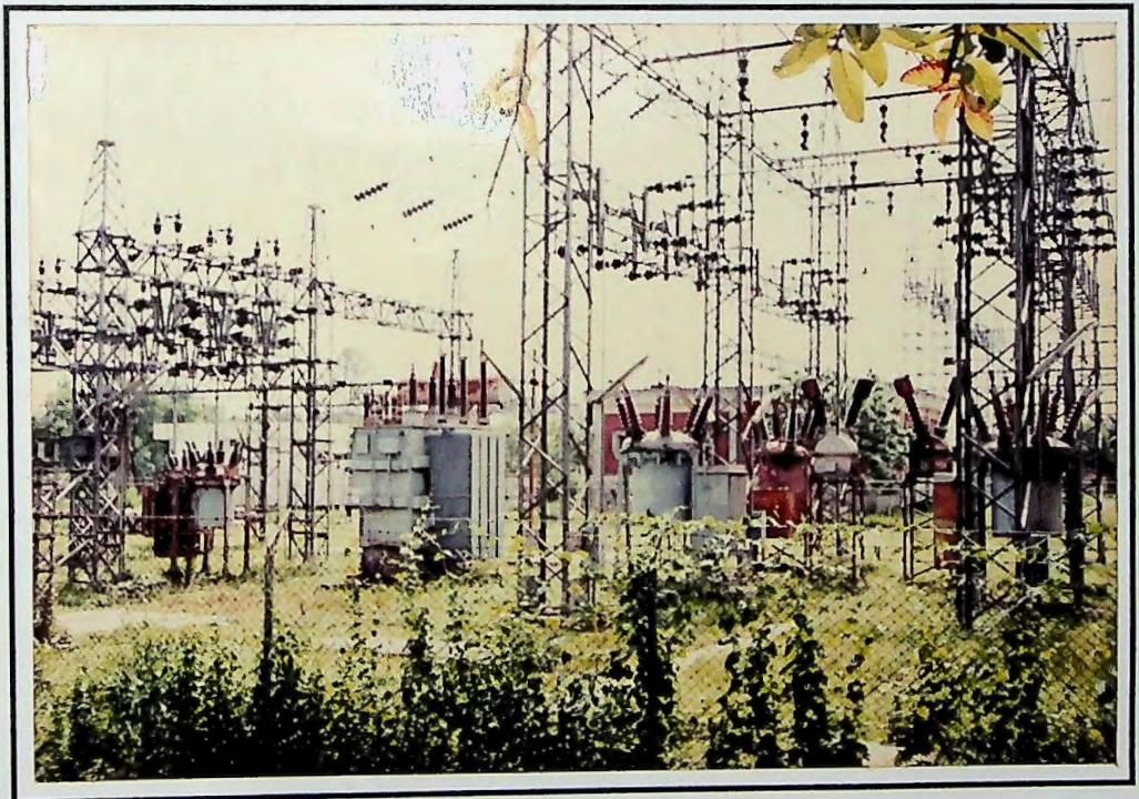
Photograph 3- Power Grid Line of Rajshahi Power Generating Station.
