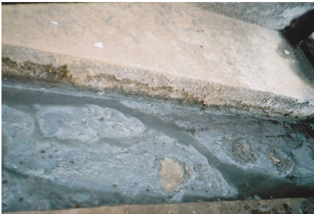
Photograph -11: Fleshings blocking the drain at Hazaribagh Bazar area
