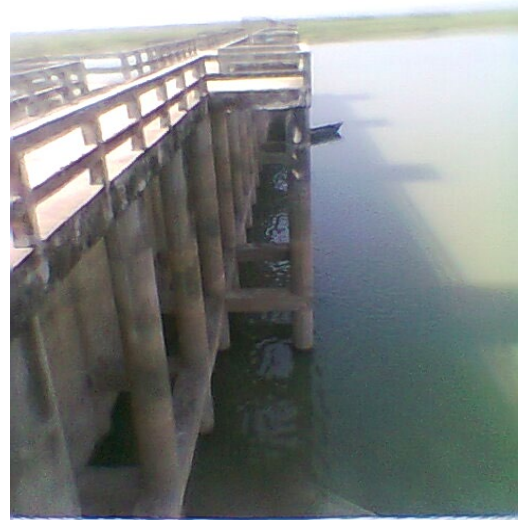
Flood Protection Measure of Haat Area
