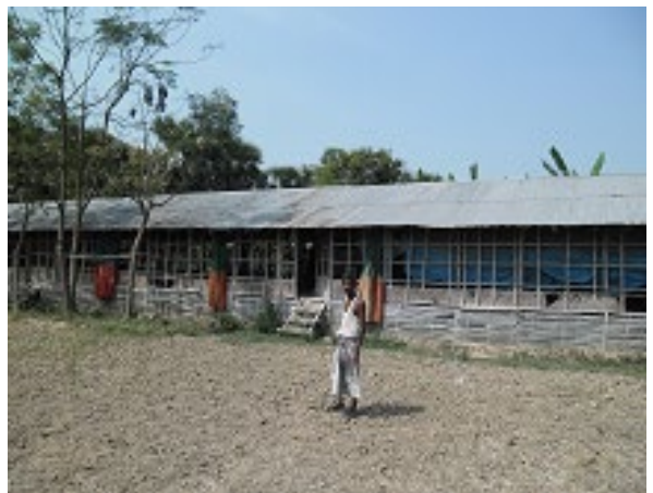
F Absence of boundary wall at Motihar farm
